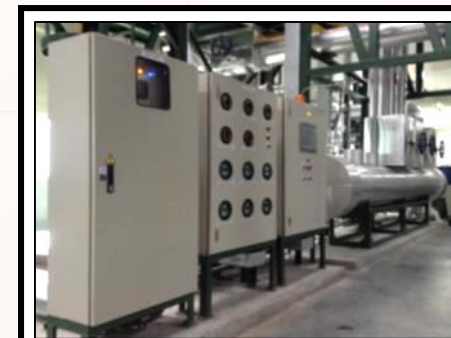
Steam Buffer Tank
